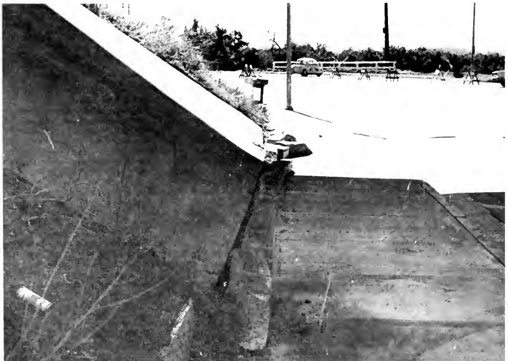
Photo 4. Concrete curbs broken by lateral movement of slope paving during fill movement.
